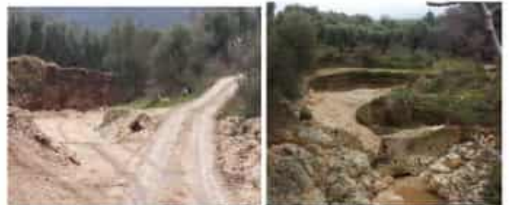
Foto 3-4 – Torrente Antonino; erosione and flood effect upstream village of Carpino (Gargano)
